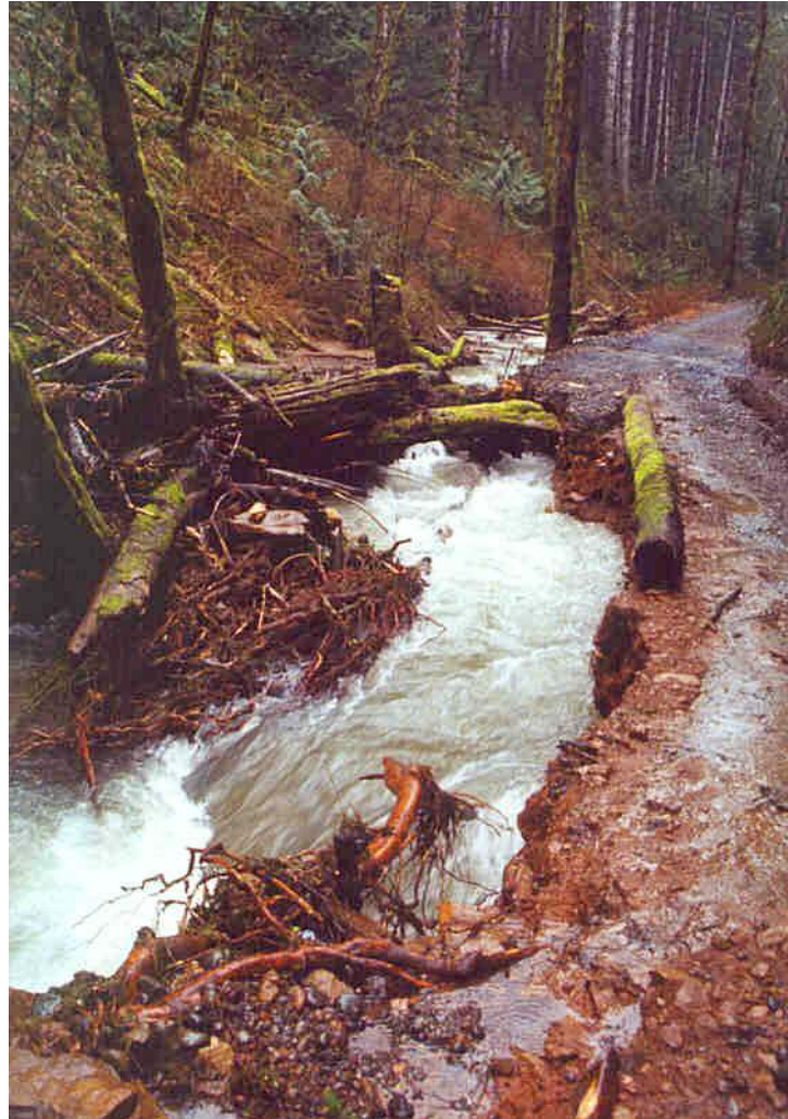
Photo 3. A debris dam on Oliver Creek formed during the 12/28/98 storm and diverted flood discharge onto Oliver Creek Road, stripping road gravel and eroding part of the compacted road bed. The clay mineralogy of this road bed material is illustrated in Figure 18B. Formation of such dams is a natural occurrence in streams with large woody debris and the associated channel diversion results in significant erosion.
